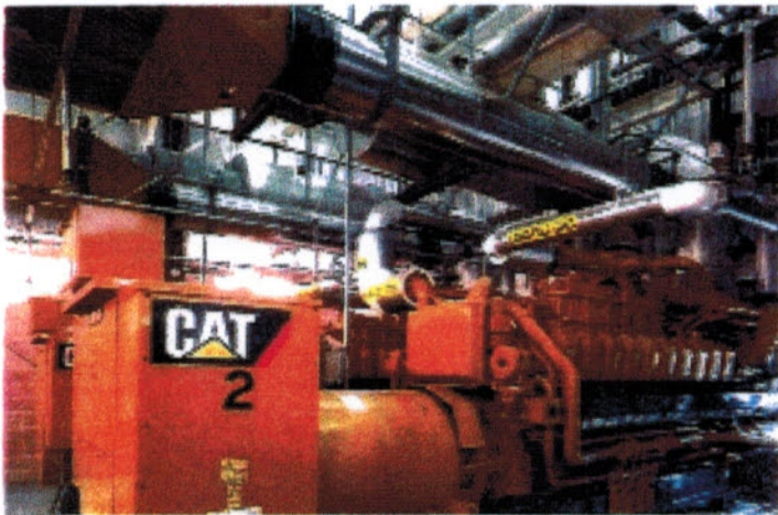
Power Generating Center
